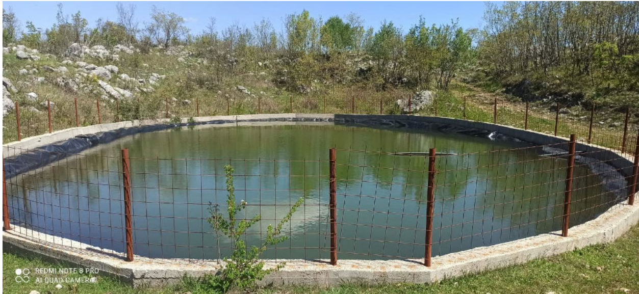
Figure 7-1: An existing water intake structure (captation basin)
